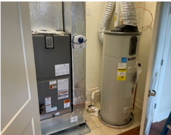
iHPWH (right) installed in a mechanical closet
