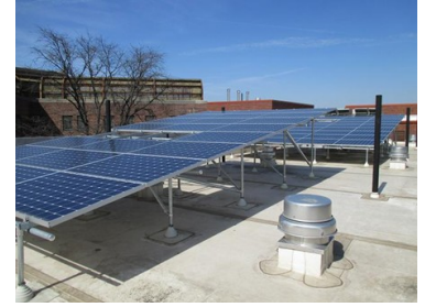
Rooftop Solar PV Panels
