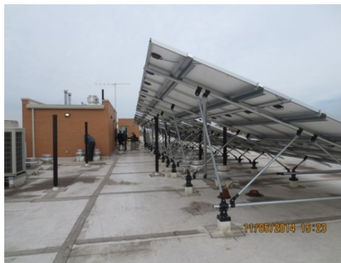
Solar PV System
