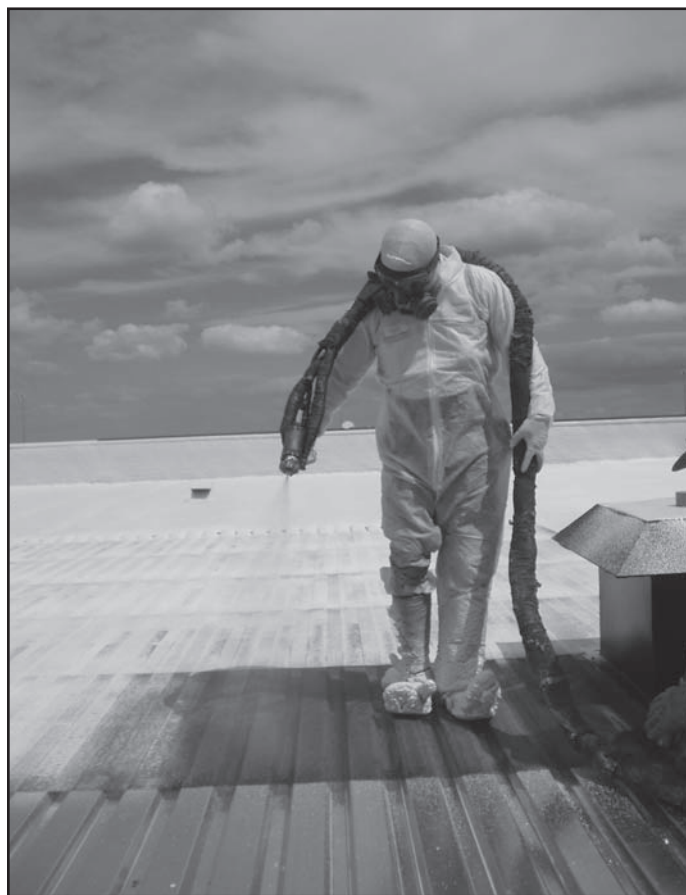
Figure 12. Installer of spray foam for a roofing application shown in full personal protective equipment. Photo courtesy Richard Duncan, Ph.D., P.E. and Spray Polyurethane Foam Alliance (SPFA).
