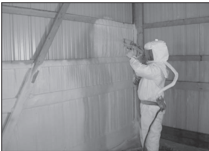
Figure 10. Closed-cell SPF insulation applied inside a metal clad building. Photo courtesy Richard Duncan, Ph.D., P.E. and Spray Polyurethane Foam Alliance (SPFA).
