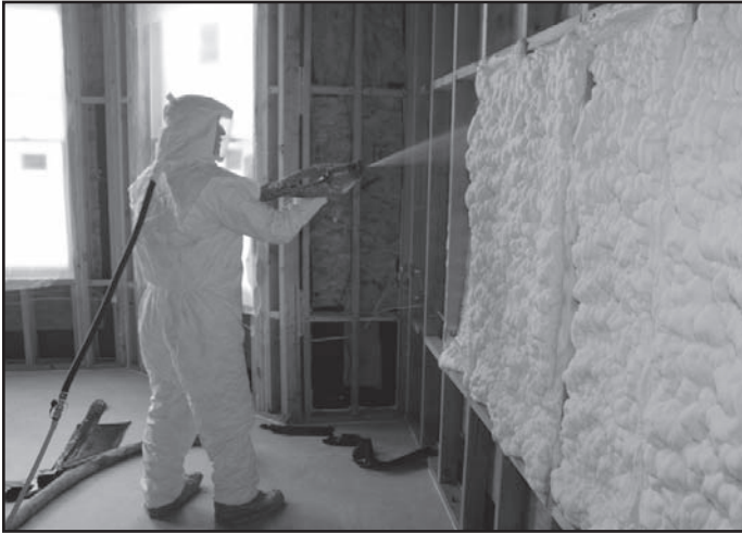
Figure 11. Installation of spray foam insulation – wood frame walls. Photo courtesy Richard Duncan, Ph.D., P.E. and Spray Polyurethane Foam Alliance (SPFA).
