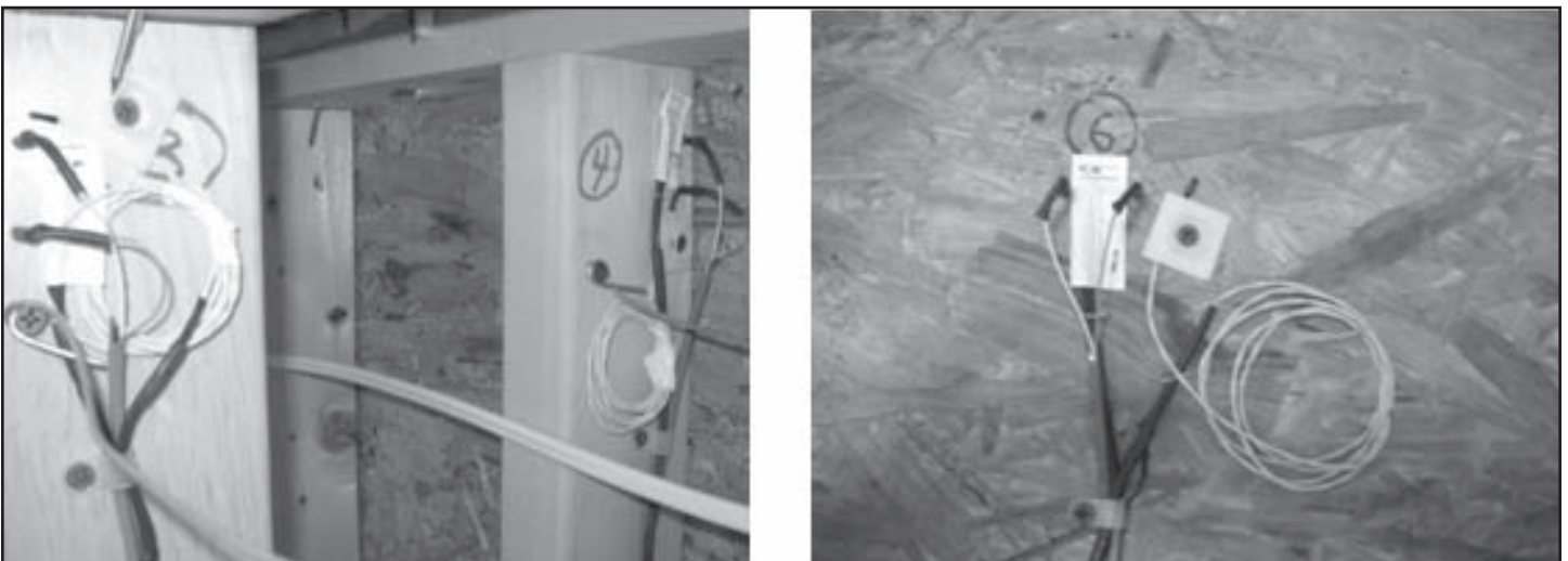
Figure 6. Typical cluster of temperature, relative humidity, and moisture content sensors. Photo courtesy Steven Winter Associates, Inc.
