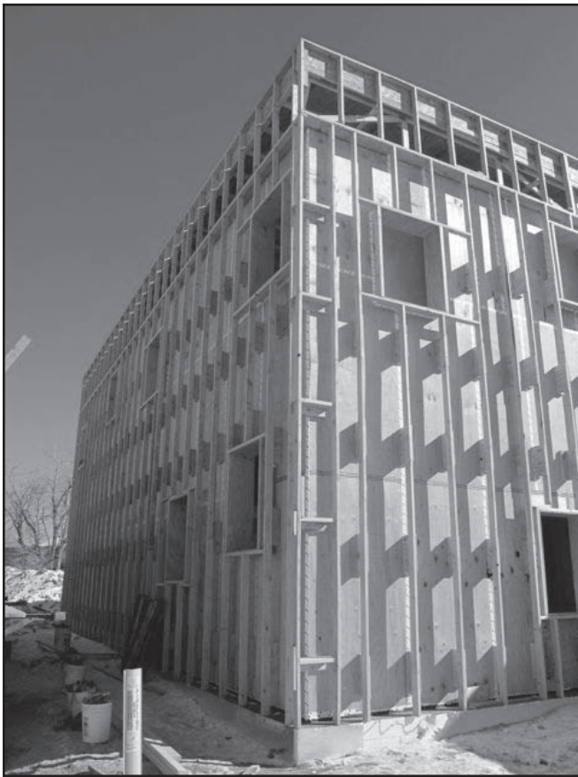
Figure 3. Project at rough framing. The Larsen Trusses are in place forming a 9" cavity for cellulose insulation forming the primary thermal envelope. The plywood air barrier can be seen behind the trusses fully taped. Image courtesy Mojarrab Stanford Architects (MoSA).
