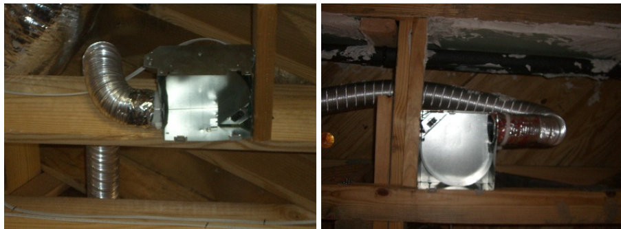
Figure 1. Common Installation Issues: Immediate bends after exhaust fan and 180° turns due to poor planning during installation.
