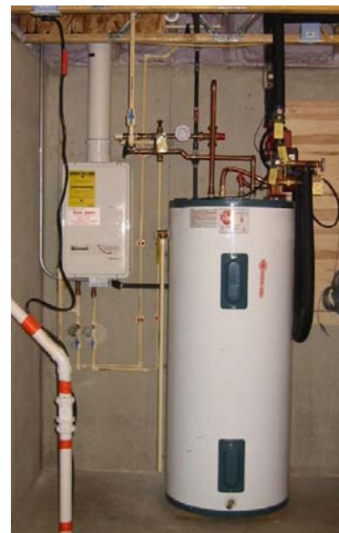
Fig. 3: Auxiliary tankless gas water heater and solar storage tank in basement of Madison home.
